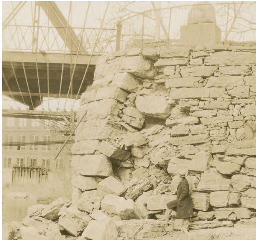
Figure 22. Detail of McAllister photograph taken ca. 1926 of a failing abutment on the iron bridge (built ca. 1885) showing gate control of the mill in the background (Lois L. McAllister Photographs Collection, Box A19, Folder 09, Item 07, Silver Special Collections, Billings Library Annex, University of Vermont, Burlington, Vermont). Note the head gates in background and the monument to Allen's fort on top of northeast bridge abutment ( Burlington Free Press July 31, 1914; February 19, 1926).
