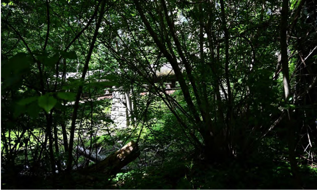
Figure 21. June 2024 view of the remains on the large diameter steel/iron penstock (VT-CH-1298), looking northwest.
