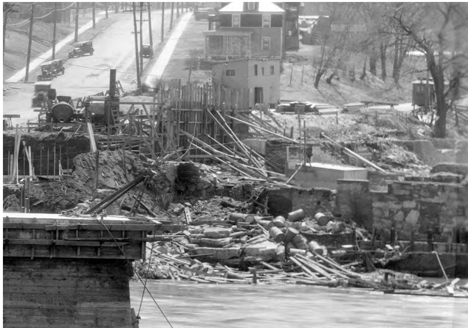
Figure 55. Detail of a view showing the old mill foundations during the 1928 bridge construction (Lois L. McAllister Photographs Collection, Box A19, Folder 13, Item 05, Silver Special Collections, Billings Library Annex, University of Vermont, Burlington, Vermont).
